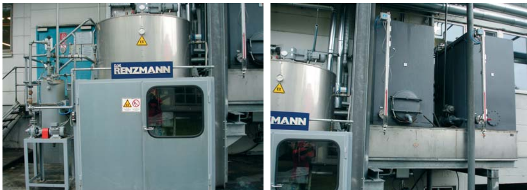
Left: Due to limited space in the washing room, the Rotomax distillation unit was installed outside the room.
