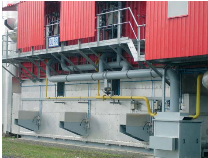
RTO exhaust air cleaning system.
